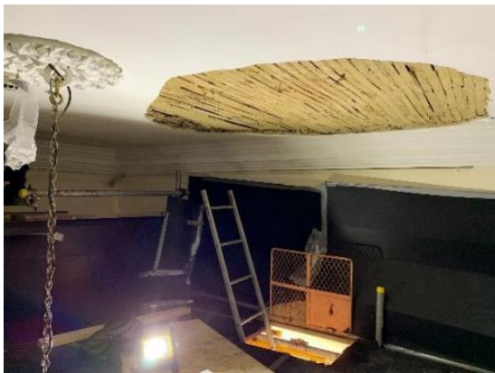
Area of fallen plaster
